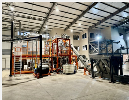
Commissioned VacuDry® 1 500 plant
