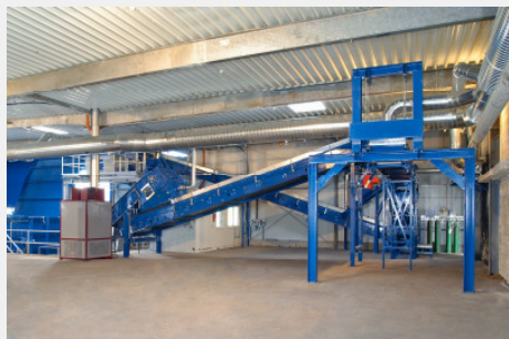
Position inside the building with conveying systems
