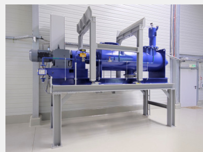
Immobilisation plant, commissioning in 2009
