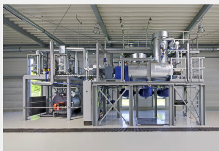
Plant „MSA-II“, commissioning in 2009
