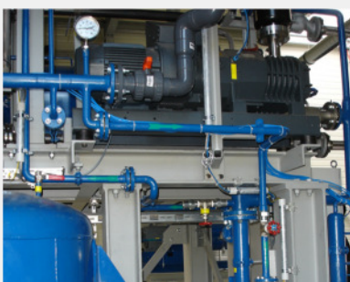
Detail of plant „MSA-II“, vacuum system
