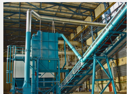
Preparation and feeding system of the plant
